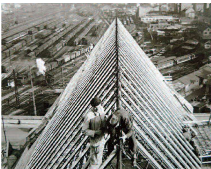
Rys. 1. Konstrukcja dachu z lekkich kratownic, wykonanego w 1950 r. w Monachium [66] Fig. 1. Roof construction with light trusses, made in 1950 in Munich [66]
